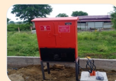
ELECTRIC NETWORK WITH TRANSFORMER
