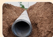
SEWAGE PIPE LINE
