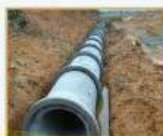
SEWAGE PIPE LINE
